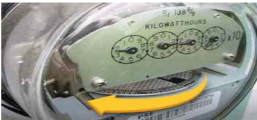
Fig.5 Net Metering [When you generate extra electricity (more than what you can use)]
